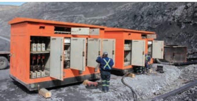
Medium Voltage Prefabricated Substation
