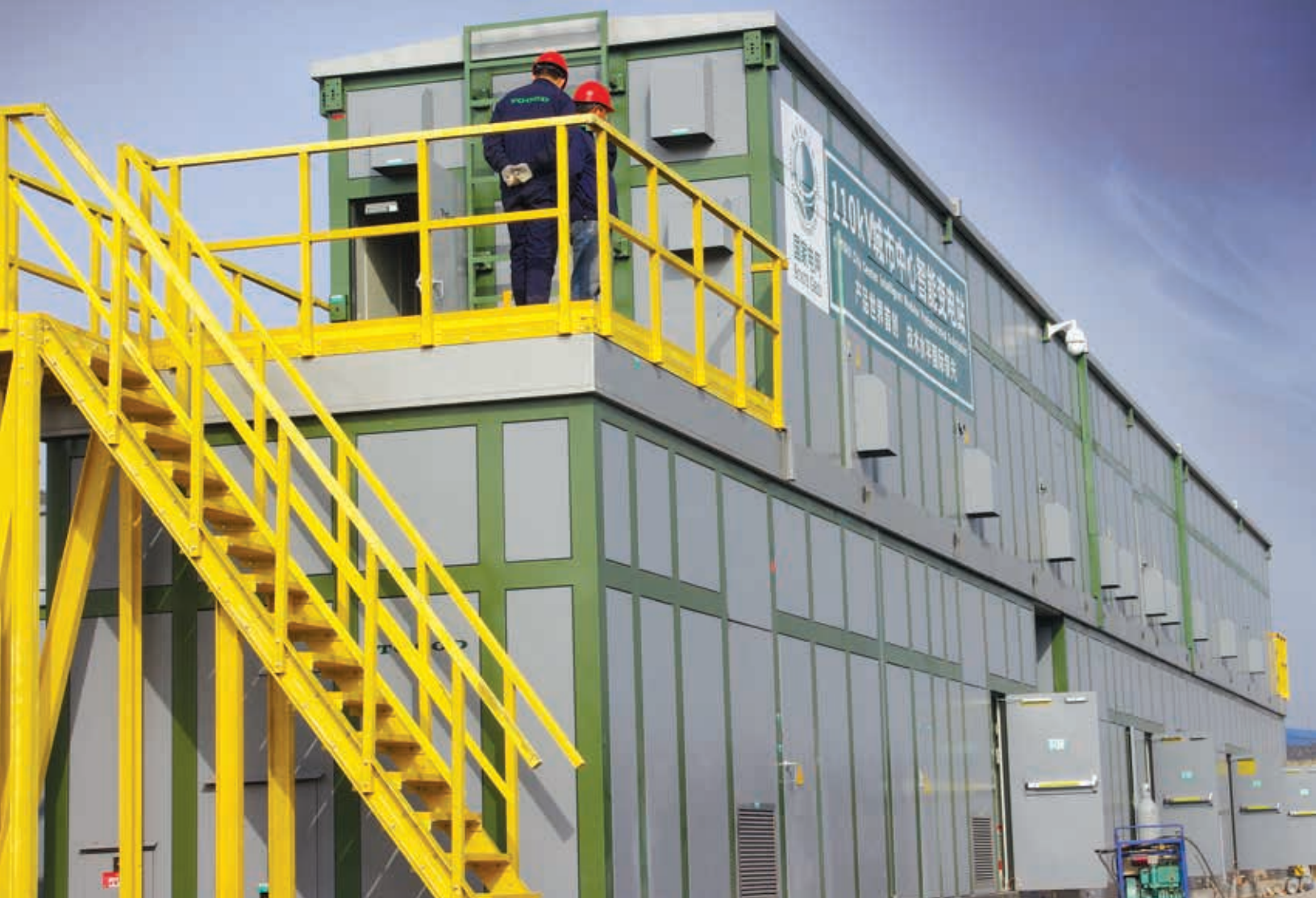
145kV Compact GIS Substation
