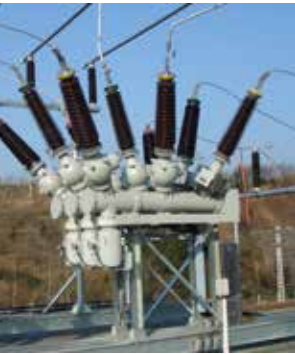
Hybrid Gas Insulated Switchgear (HGIS)
