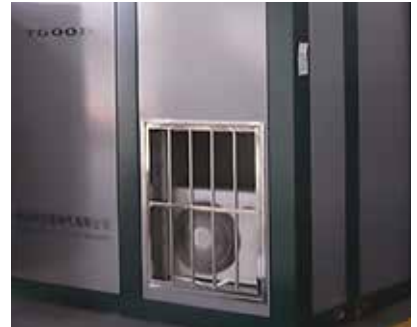
Air Conditioning Unit
