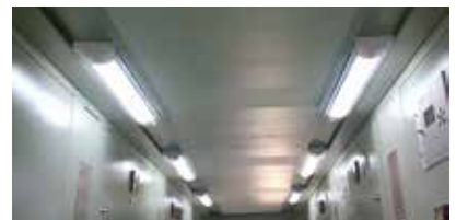
Ceiling Lighting and Sound Deadening Panels
