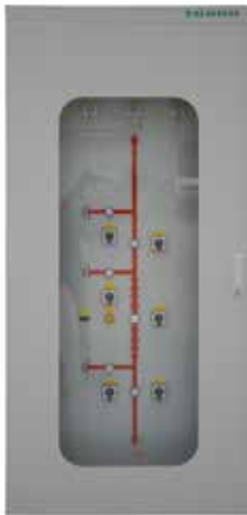
Local control panel
